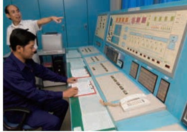
The monitoring room at the Phum Prek Water Treatment Plant in Phnom Penh, where the system is monitored around the clock.
