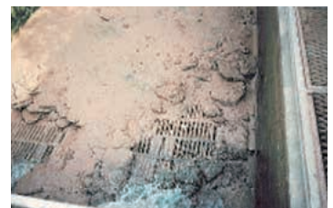
Photo from around 1993 of the neglected filtration pond at water treatment plant.
